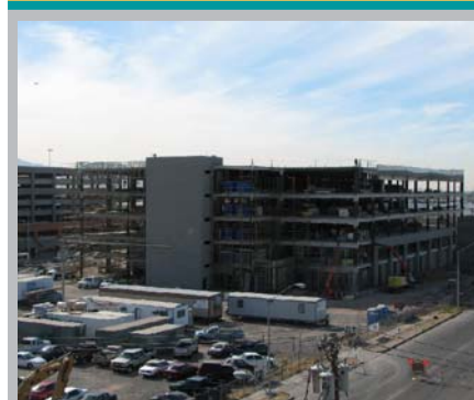
The building up a new court facility. Above is a recent photo of the construction of the new 254,300 square-foot Downtown Justice Court Center (DTJC). The Clerk's Office will have offices on the 3rd floor of the five-story building. The DTJC building is projected to be completed in December.
