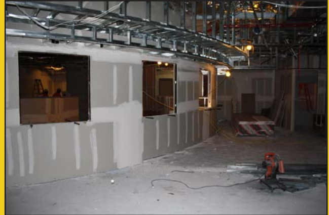
A portion of the new Filing Counter area being constructed in September.
