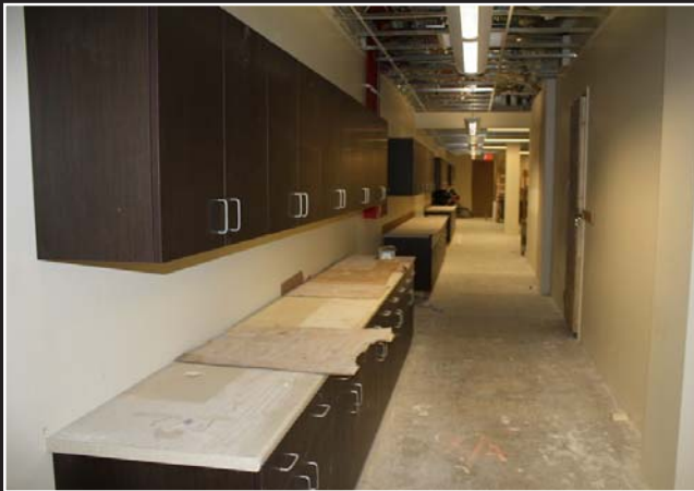
Row of storage cabinets.
