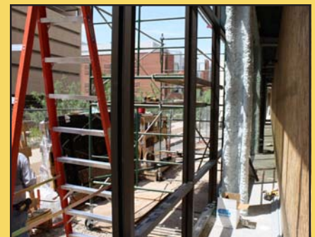
Window framing being put in place for the south side of the office.
